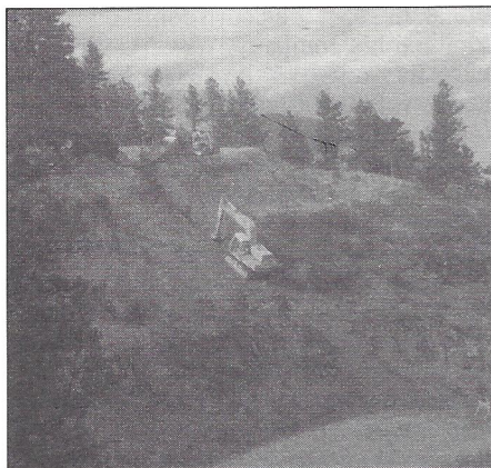
The pipeline contractor was experienced in mountain construction. The backhoe on this 65-degree slope is secured by a bulldozer-supported cable.
